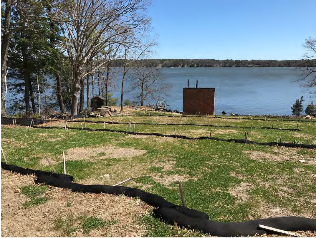
Fig 1: Upper portion of slope leading down to cable house and salt marsh restoration at the west side of the bay. Viewing east. (04-26-21)
