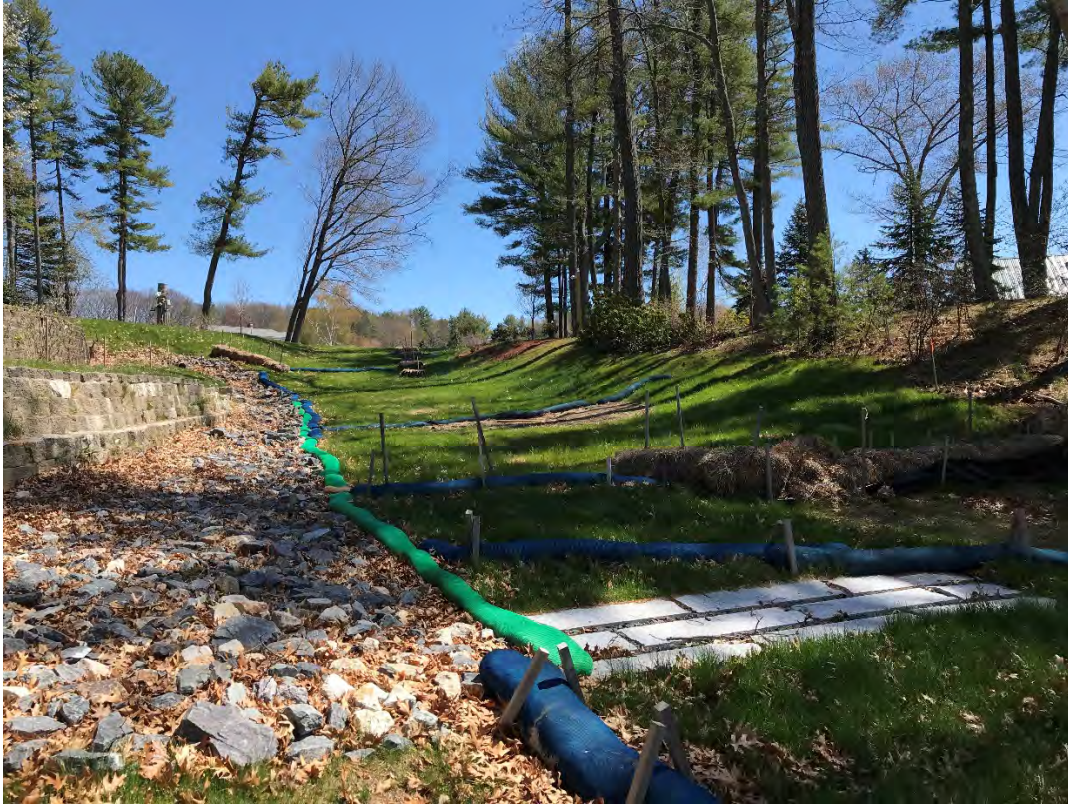
Fig 9: Slope above the manhole at Gundalow Landing/east side of the bay. Viewing east. (04-26-21)
