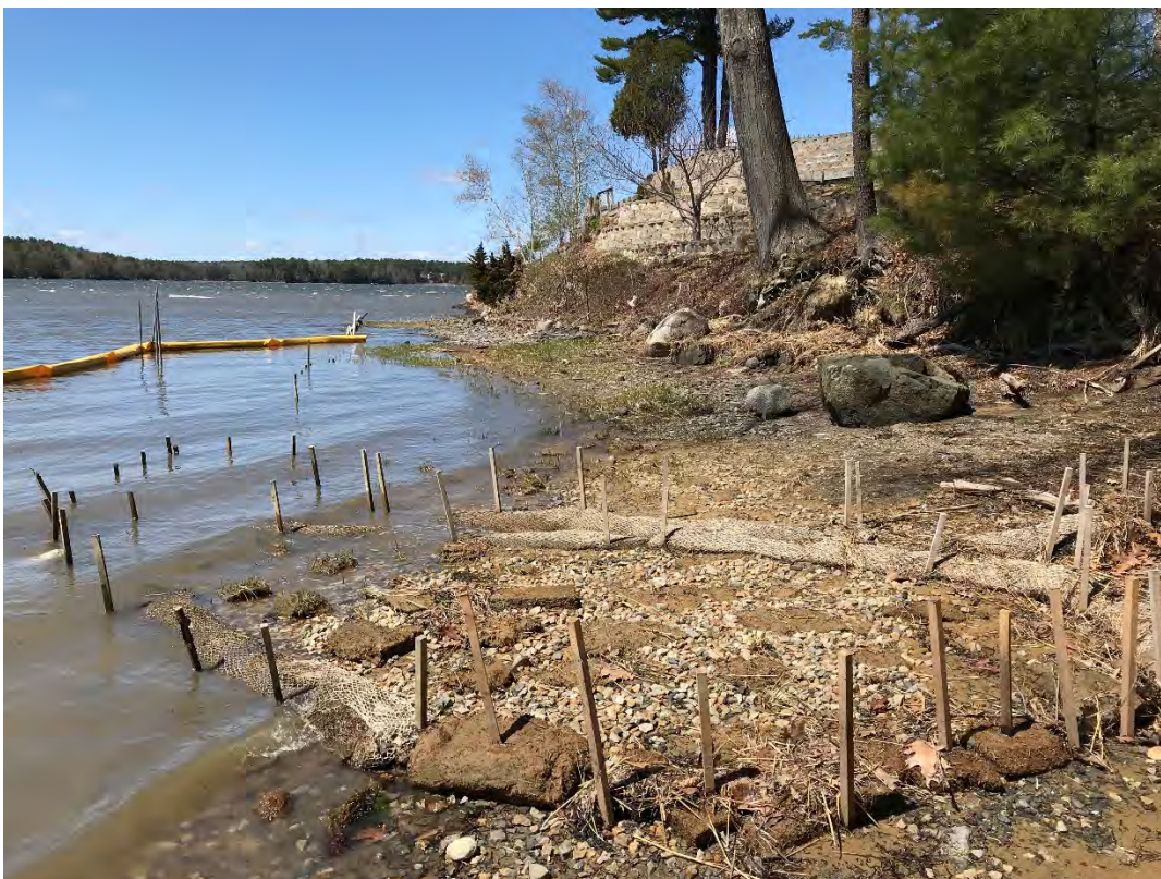
Fig 12: Salt marsh restoration at Gundalow Landing/east side of the bay. Viewing south. (04-26-21)
